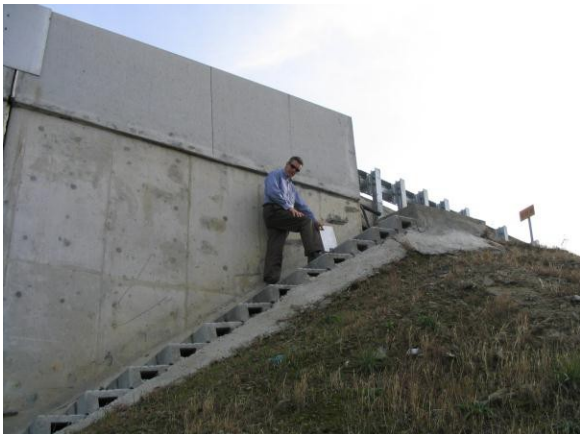
Figure 3. Bridge abutment settlement
